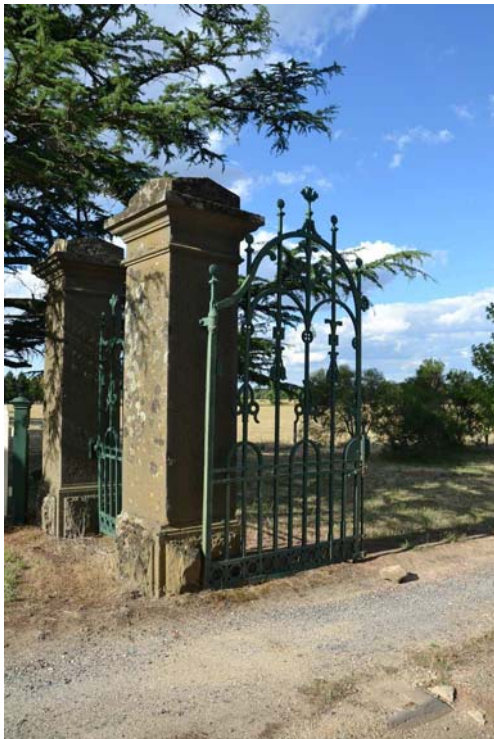
Photo 5 Pillar showing slight damage and rotation.
