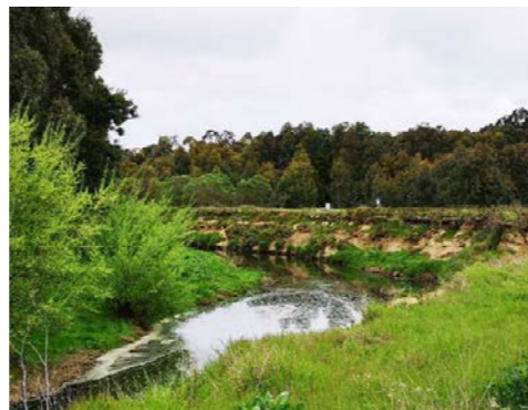
Severe erosion along the river bank
