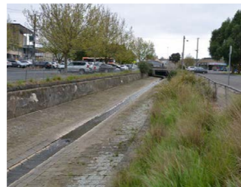
Yarrowee River channel at Anderson Street with car parking on both sides
