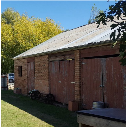
Figure 30. The same end of the Plough Inn stables after repairs, 2018 (Tripadvisor.com.au)
