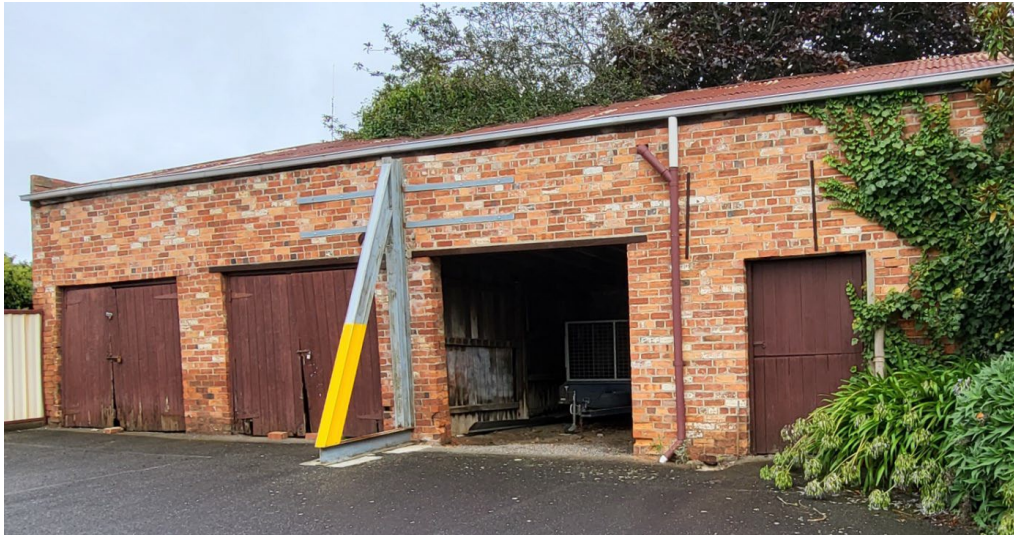
Figure 19. Southern half of the stables, with three garage doors and a divided stable door (right). (Landmark Heritage, 2023)
