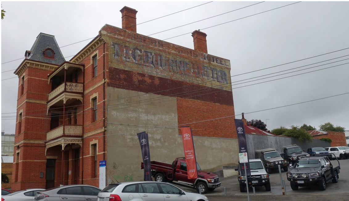
Figure 15. Hotel viewed from the north-east, with the painted signage visible at parapet level. Rising damp is visible at the base of this wall. (Landmark Heritage, 2023)
