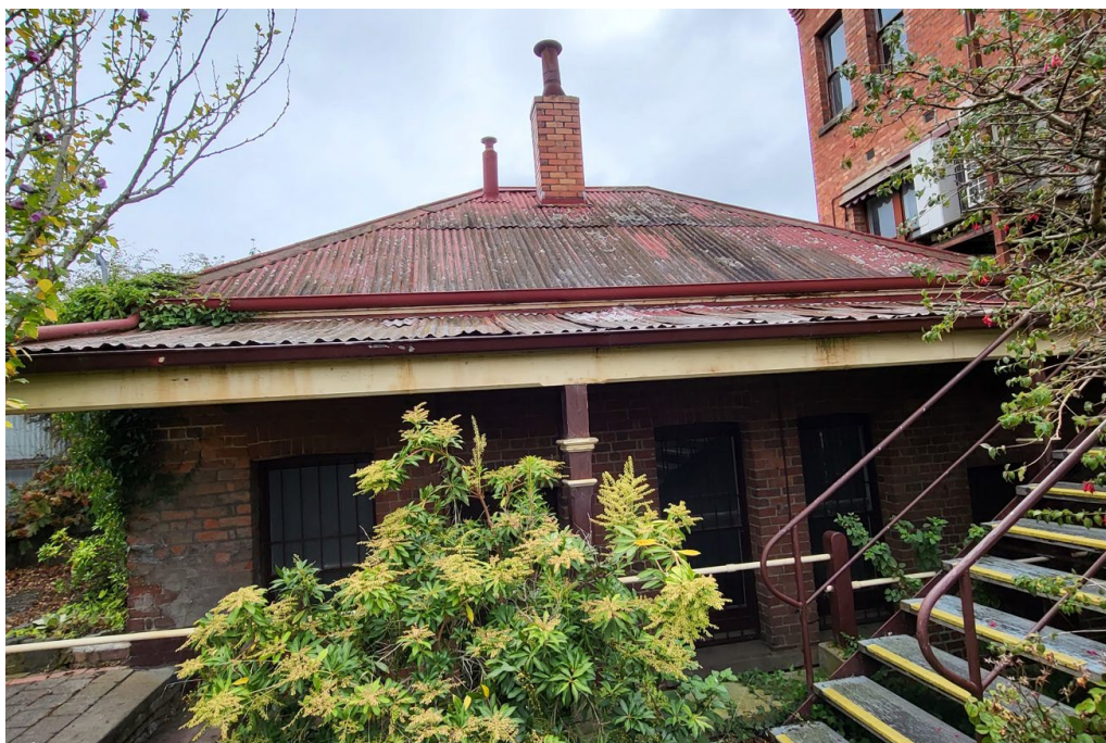
Figure 16. The kitchen, viewed from the south. A timber verandah post is visible at centre. (Landmark Heritage, 2023)
