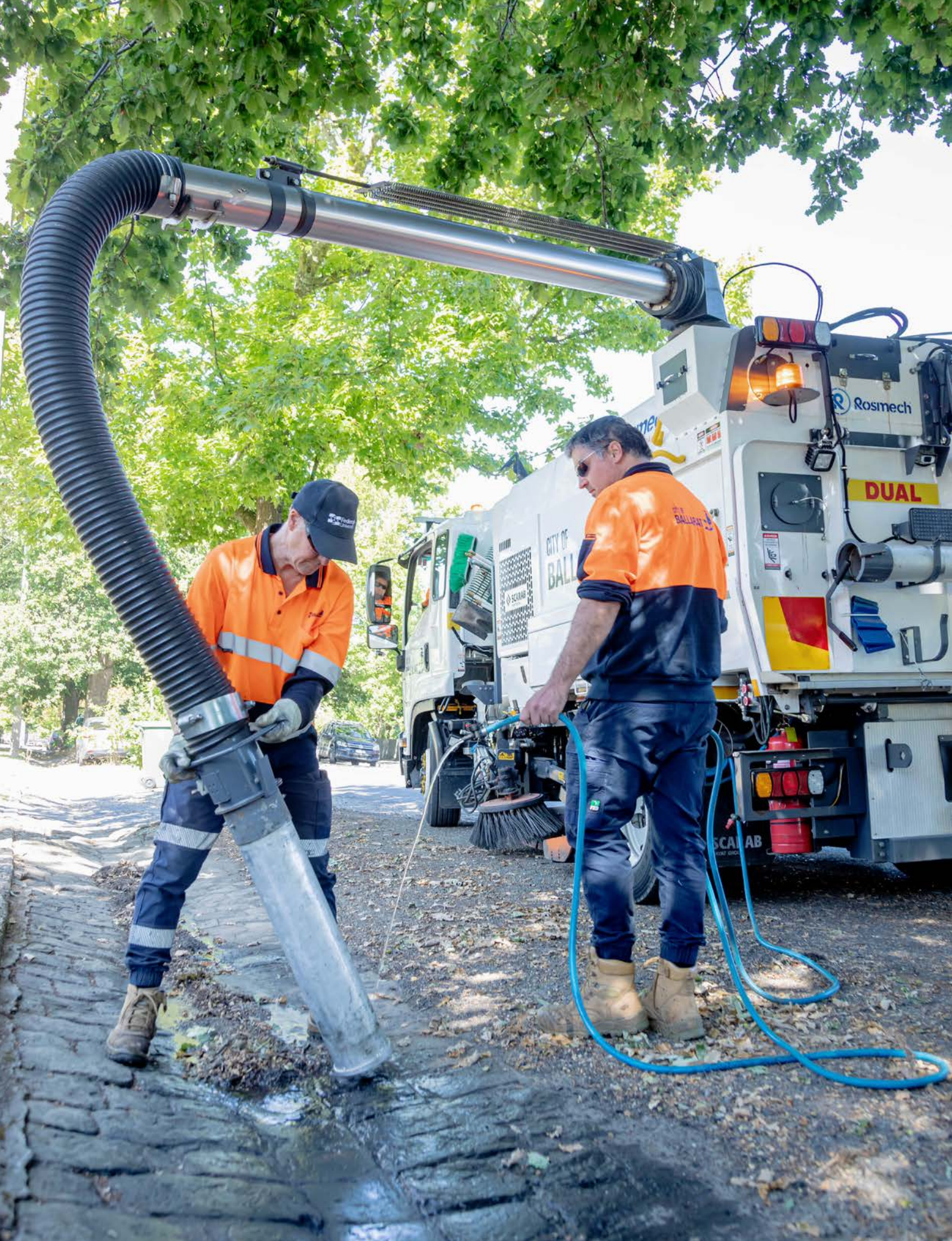
📷: Members of the City of Ballarat Street Cleaning Team at work in Durham Street, Newington.
