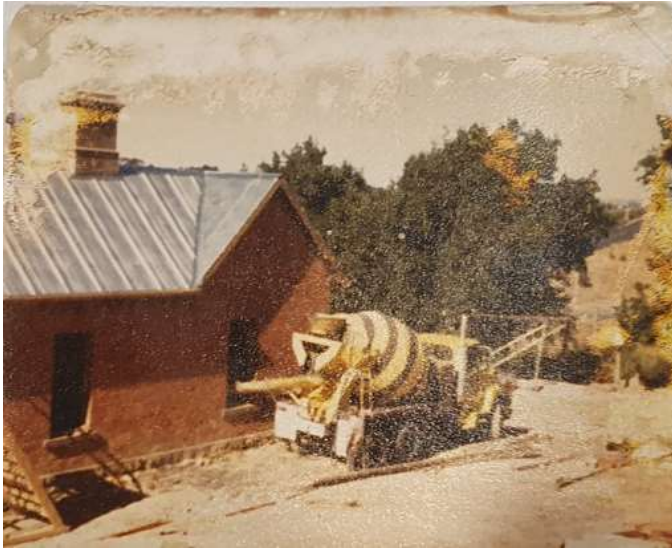
Figure 4. The former Parsonage undergoing works c1981. Note the new roofing, windows removed, and mixer pouring a concrete floor. (Collection of C & M Sargent)
