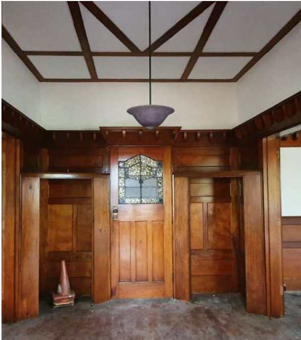
Figure 9. Entrance hall, as viewed from the front door. The door here leads to the back corridor, and is flanked by coat closets with doors removed. (Landmark Heritage, 2022)
