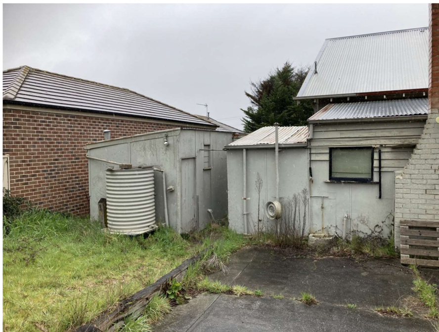
Figure 6 View to outbuilding north east of dwelling from rear yard, also showing c.1933 skillion kitchen and brick chimney.
