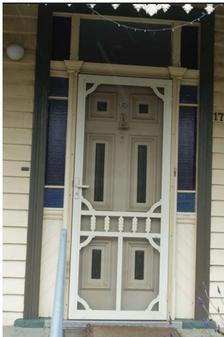
Figure 14. Original six-panel front door at No. 17. Note the pressed glass and diagonal boarding below sidelights. (Landmark Heritage 2022)
