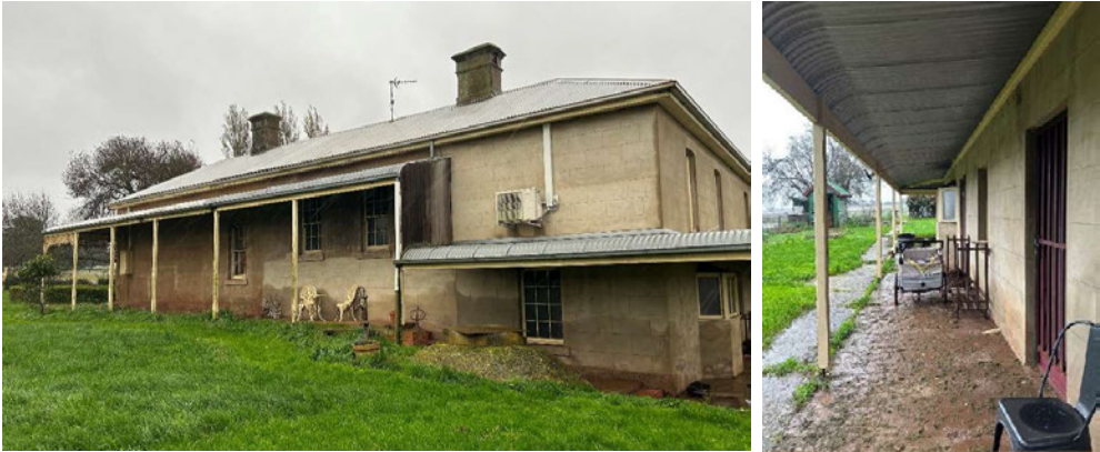
Left: The Southern elevation with colour difference shows additions over decades. Right: The Eastern elevation.
