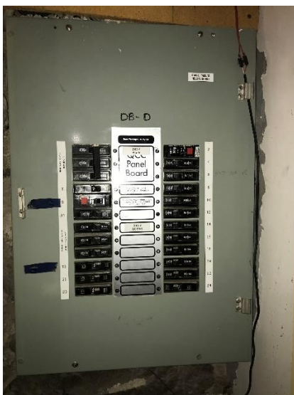
FOH Switchboard –Basement Level 1
