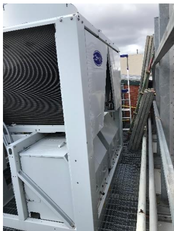
Air cooled Chiller
