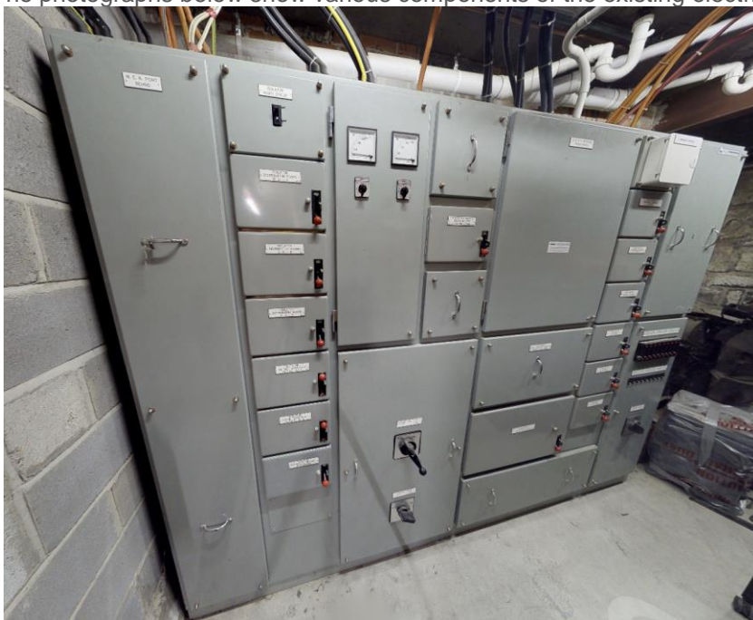
Main Switchboard – Basement Level 1
