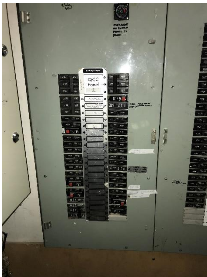
FOH Switchboard –Stalls Level 3
