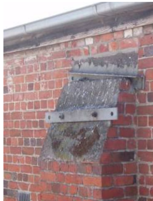
View of deterioration to pilaster
