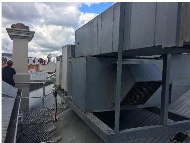
Existing Long Room air conditioning system
