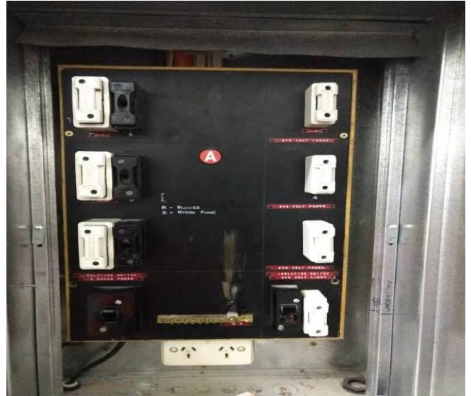
Photo 2 – Sub Basement Store 5 Zelemite switchboard
