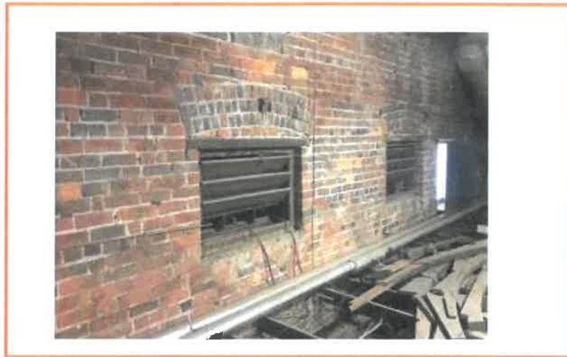
Figure 2: Existing West Wall Proposed Fire Wall in roof space (typical required upgrades)
