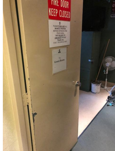
Photo 8 – Green room metal door has lead containing paint
