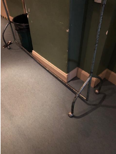
Photo 7 – Green room floor skirting has lead containing paint
