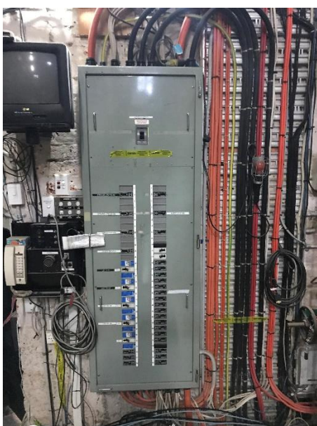
Stage Switchboard – Stalls Level 3
