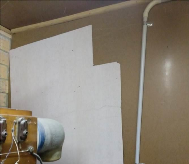
Photo 1 – Sub Basement Drum room fibro cement loose sheeting against wall
