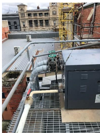
Gas fired boiler
