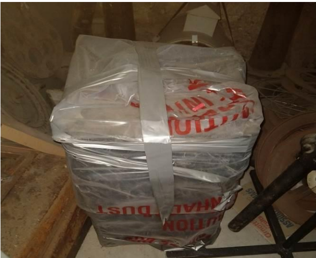
Photo 3 – Sub Basement Switch room wrapped asbestos labelled item
