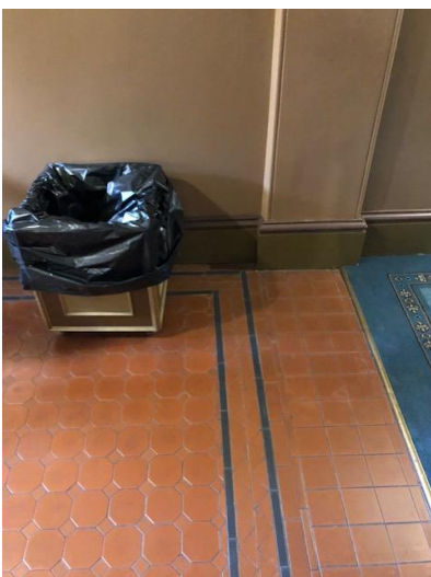
Photo 17 – North entrance lower skirting Has lead containing paint
