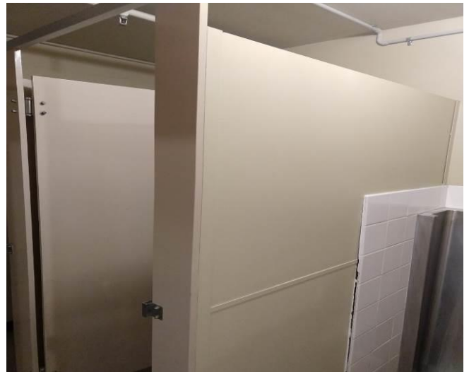
Photo 4 – Sub Basement Male WC 2 fibro cement urinal surround
