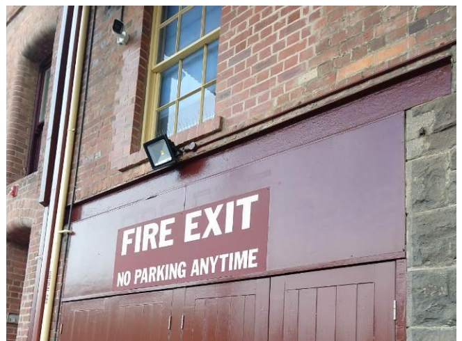
Photo 6 – Externals Auditorium fire escape fibro cement infill panels above exit doors
