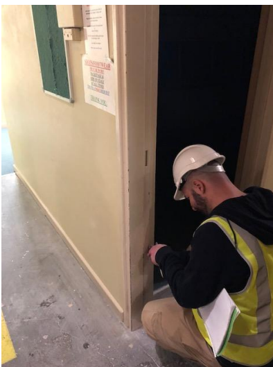
Photo 11 – Basement dresser door frame has lead coated paint
