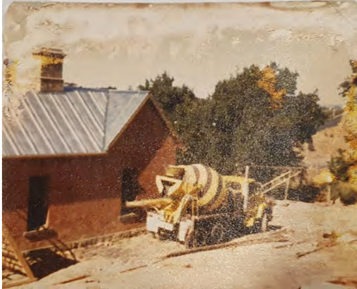
Figure 4. The former Parsonage undergoing works c1981. Note the new roofing, windows removed, and mixer pouring a concrete floor. (Collection of C & M Sargeant)
