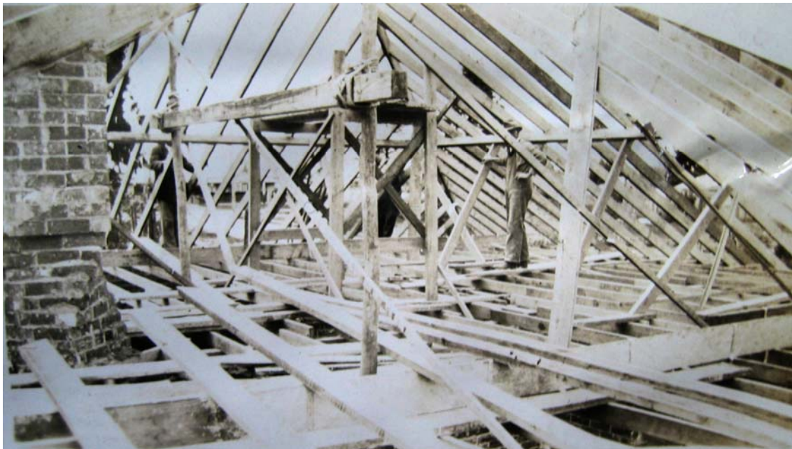
Figure 2.23: Construction of roof structure, possibly at the “All Electric Home” at 7 Colpin Avenue, 1933. Source: Bruce and Mary Green collection provided by Jennifer Burrell, Colpin Avenue, June 2005.
