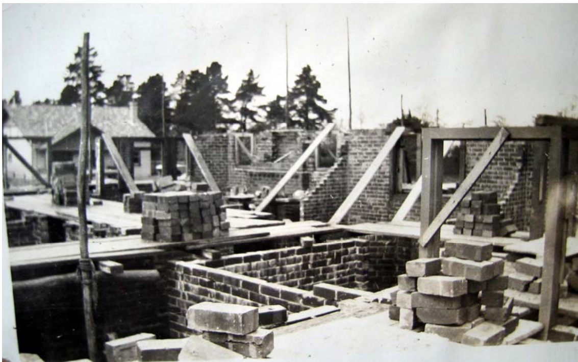
Figure 2.21: “All Electric Home” at 7 Colpin Avenue under construction in 1933, showing brick base walls supporting timber floor structure. Source: Bruce and Mary Green collection provided by Jennifer Burrell, Colpin Avenue, June 2005.
