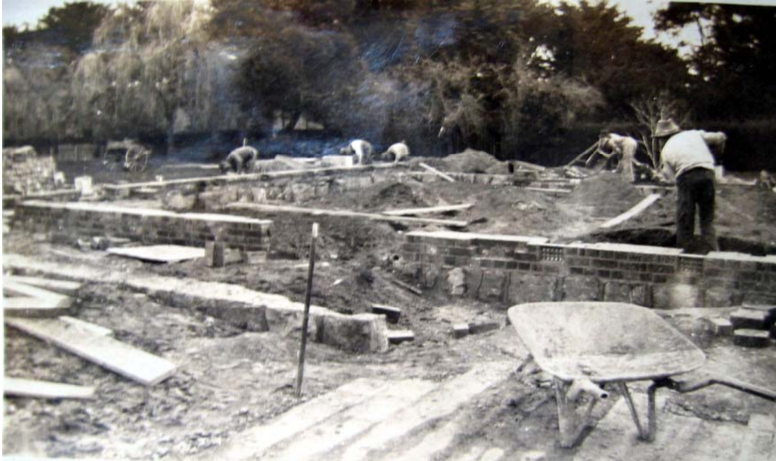
Figure 2.20: Possibly the “All Electric Home” at 7 Colpin Avenue under construction in 1933, showing the foundations and brick base walls with terra cotta subfloor vents installed. Source: Bruce and Mary Green collection provided by Jennifer Burrell, Colpin Avenue, June 2005.
