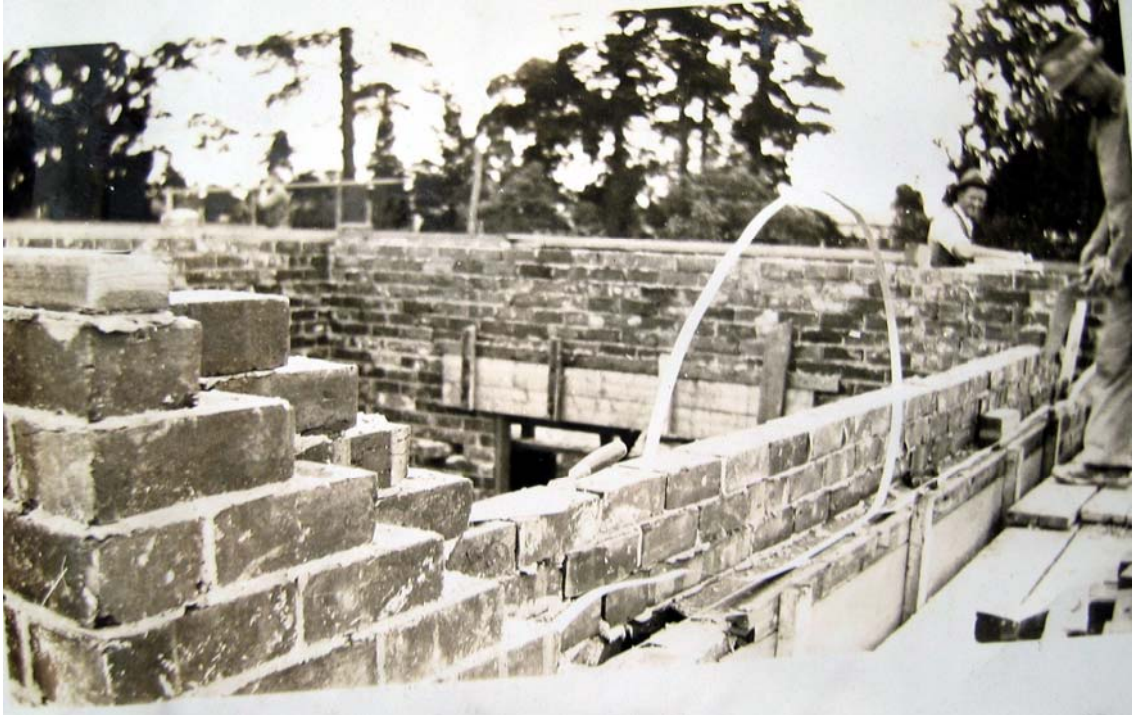
Figure 2.22: Detail of cavity brick wall construction, possibly at the “All Electric Home”, 7 Colpin Avenue in 1933. Source: Bruce and Mary Green collection provided by Jennifer Burrell, Colpin Avenue, June 2005.
