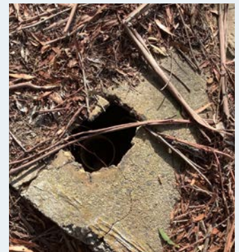
4. Damaged septic tank. (Odours, mosquitoes, water ingress leads to failure)
