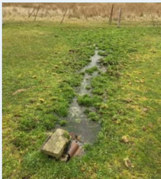
1. Absorption trenches failing. (aboveground discharge, mosquitoes)
