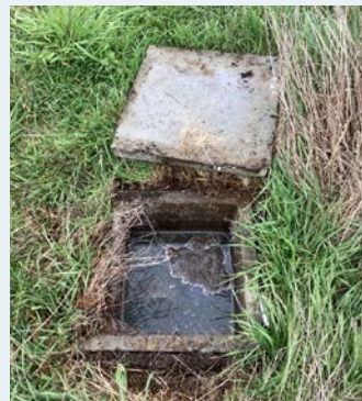
2. Solids in distribution box. (potential for system blockage)
