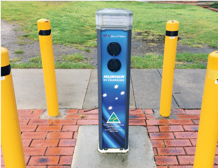
EV charger in Buninyong
