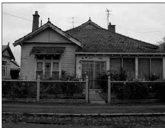
The aluminium windows of this verandah enclosure do not contribute to the significance of this Heritage Place
