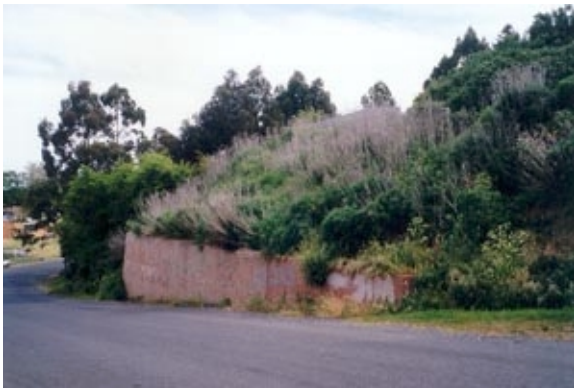
Figure 67. Weed infested road embankments.
