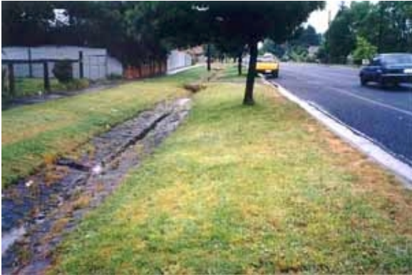
Figure 2. Multiple drainage treatment (traditional drain and modern gutter treatment) in Latrobe Street.
