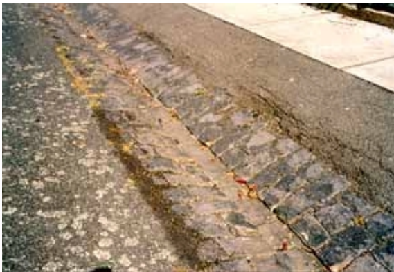
Figure 8. Bluestone pitcher spoon drain gutter with bitumen edge replacing kerb in Exeter Street.
