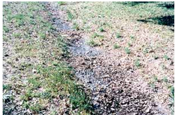
Figure 13. Open earth (unformed) drain in Russell Street.
