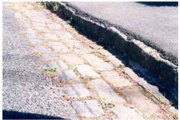
Figure 7. Bluestone pitcher invert channel gutter with bluestone pitcher kerb in Little Clyde Street.
