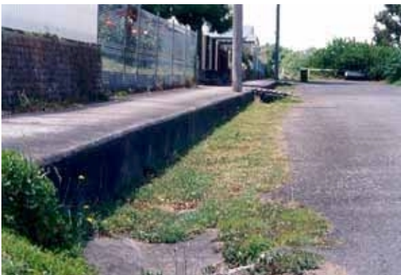
Figure 14. Retained footpath forms road edge at the southern end of Lyons Street South.
